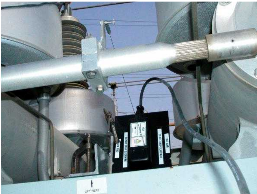
String Transducer on ABB 72PM Circuit Breaker
